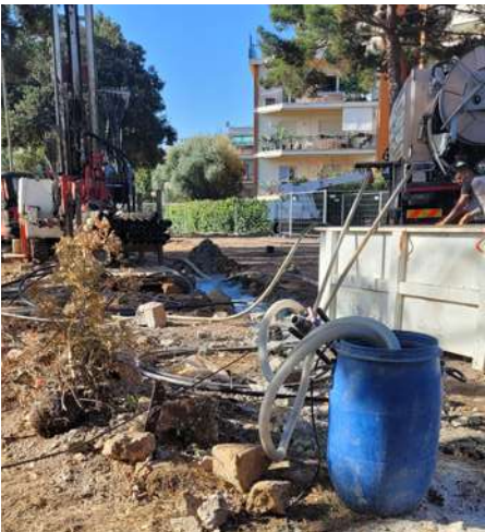
ENHANCED GROUND RESPONSE TEST- ROMA (RM) 350kW
